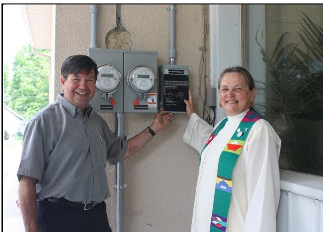
As Stan Armstrong and Rev. Marg Smith of Keswick United Church ceremonially flip the switch, the church becomes the first in town to go solar.
